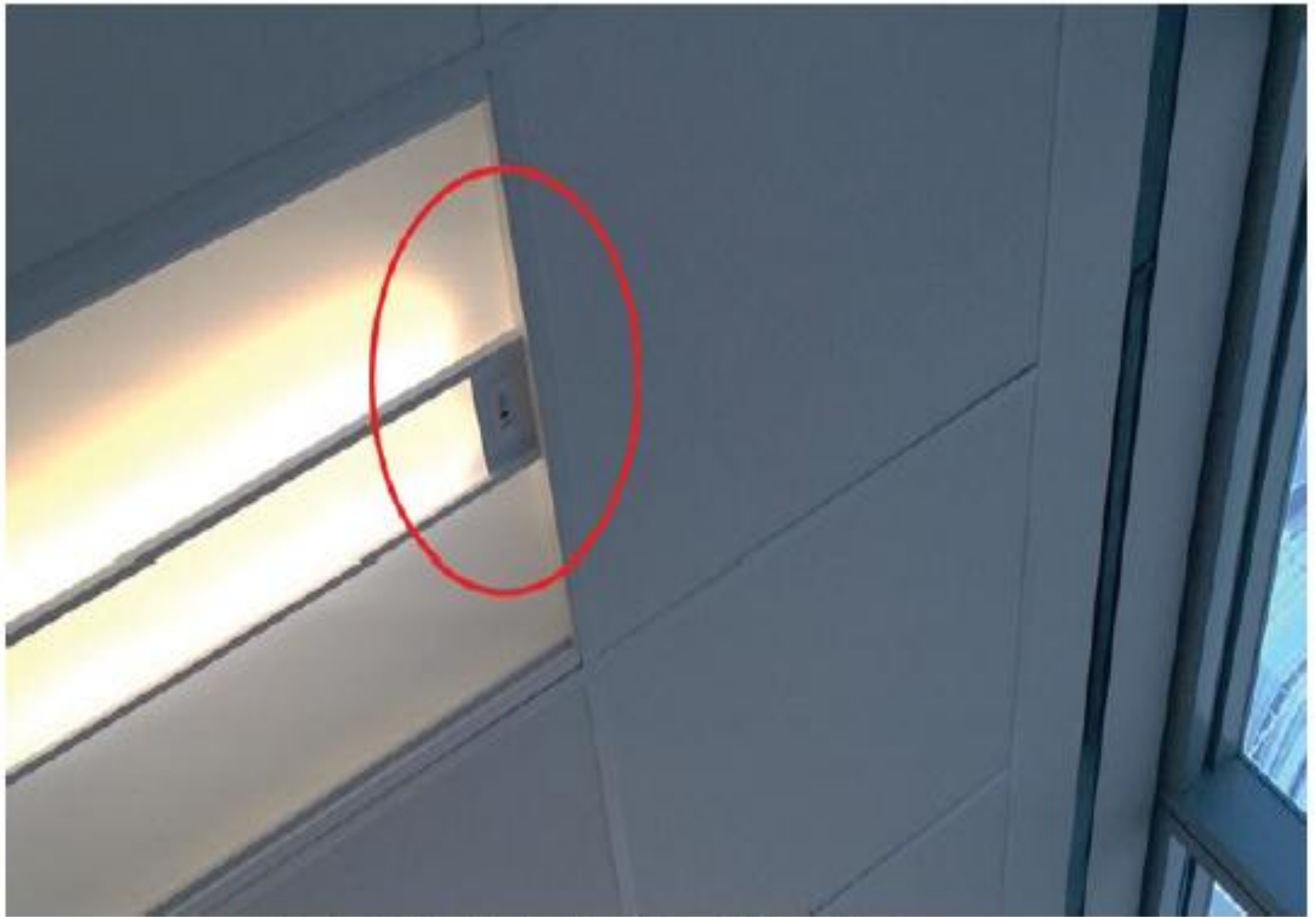
Figure 1-9 An LED Digital Ceiling Light with Occupancy Sensor
